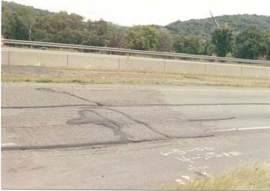
Figure 4-9: View of mining induced subsidence on I-70, east of Washington, Pennsylvania.
