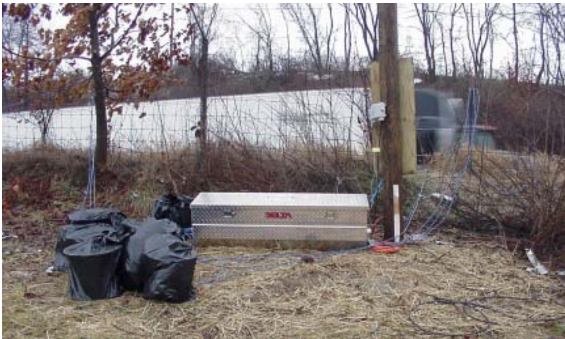
Figure 4-11: View of the portable steel enclosure hosting the datalogger and multiplexer, I-70, Pennsylvania.
