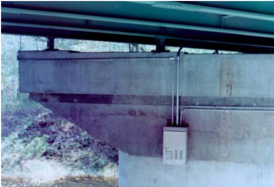
Figure 2-8: Enclosure housing the acquisition system, installed on the west side of pier No.2 of the S.R.62 bridge over the Little Blue River, Crawford County, IN.
