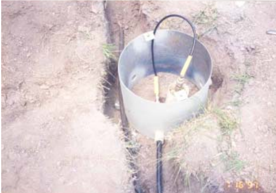
Figure 4-14: View of the horizontal lead cable, linking the TDR cable to the data acquisition system, I-70 Cambridge, Ohio.
