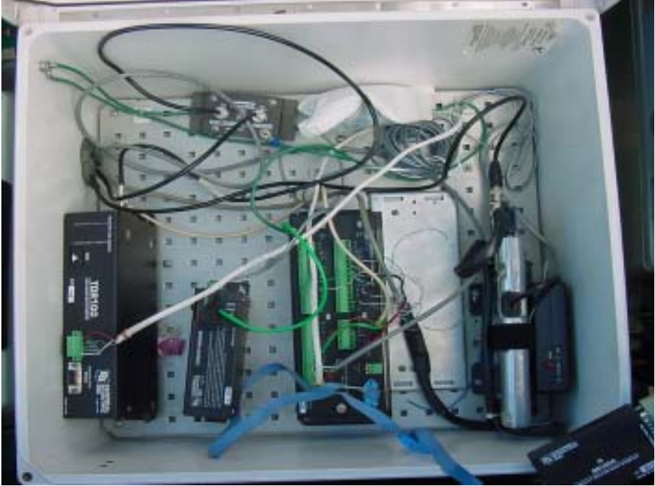
Figure 4-7: View of the remote data acquisition system installed at SR. 66, FL, based on a TXT 1502 TDR pulser (Left) and a CSI CR10X datalogger (right).
