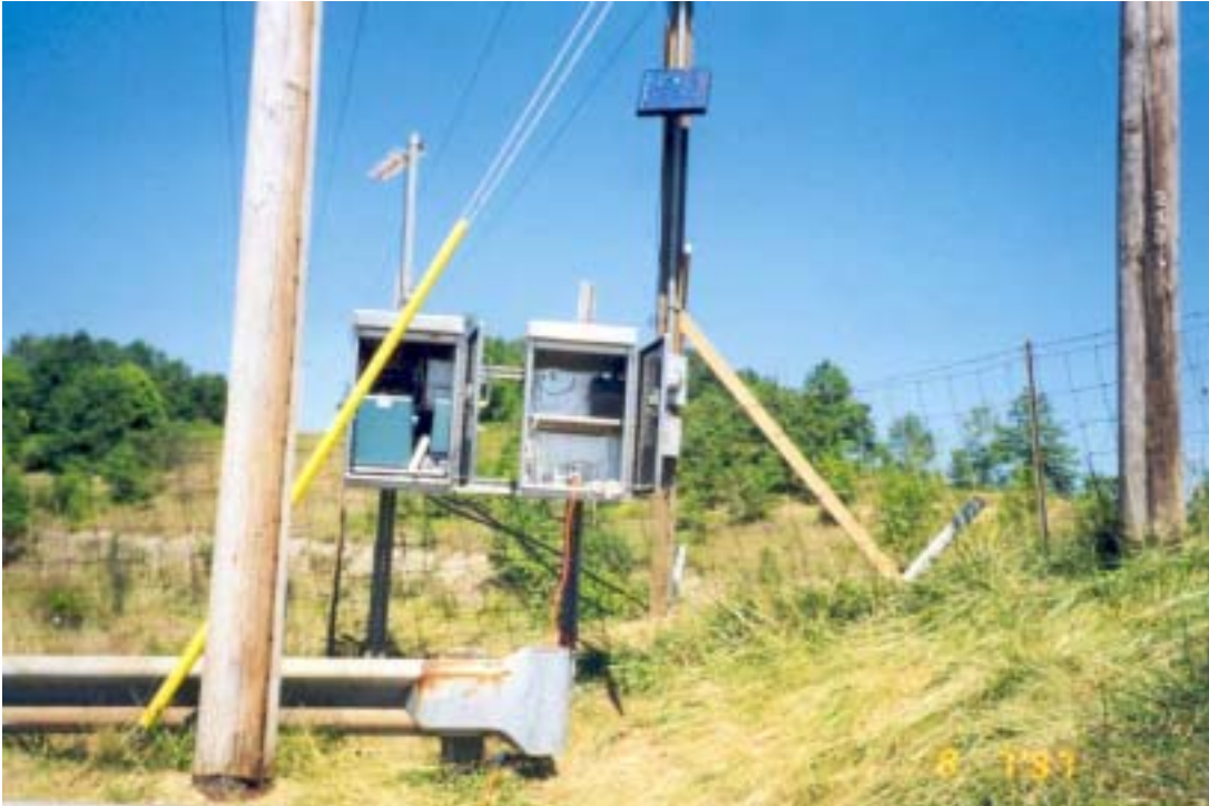
Figure 4-15: View of the enclosures hosting the first data acquisition system based on Tektronix 1502 pulser, I-70, Cambridge, Ohio.
