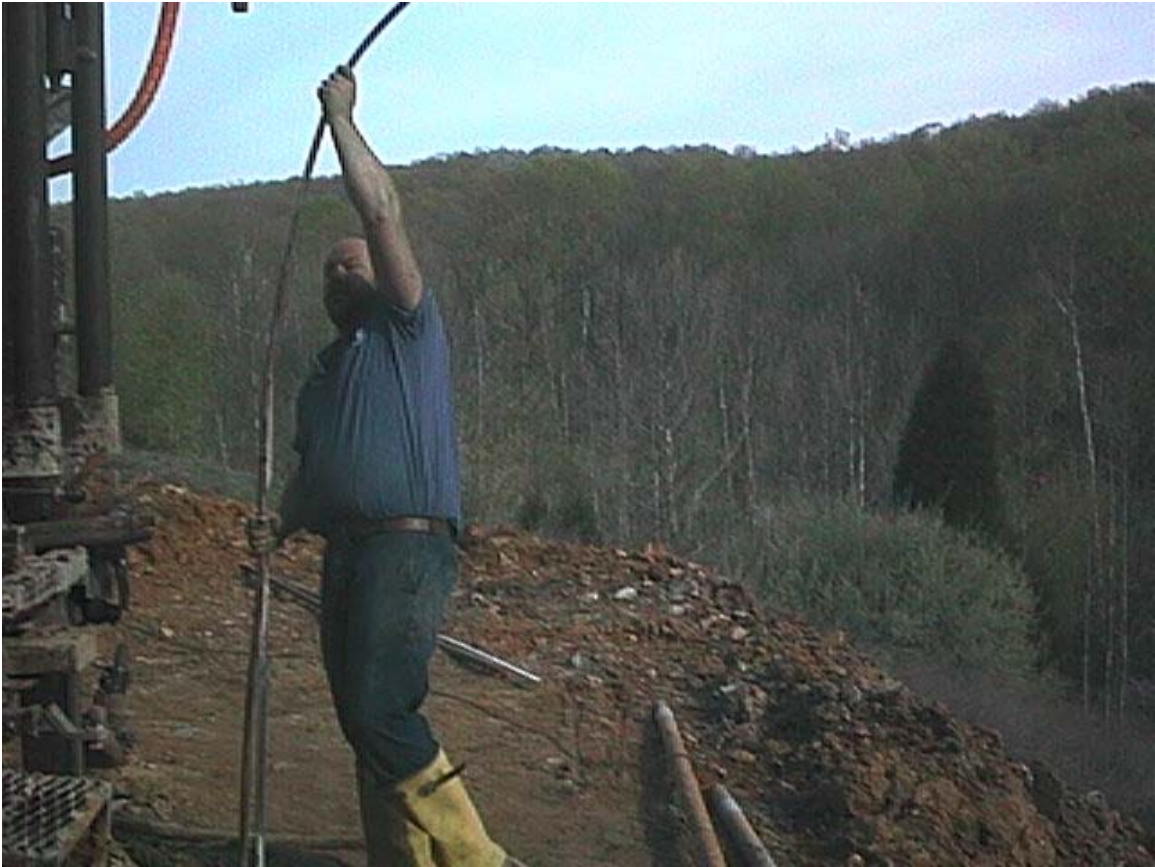
Figure 3-12: Lowering of the solid aluminum cable in open hole B-1-TDR through the hollow stem auger, bridges on I-64 over the Little Blue river, Crawford County, Indiana.
