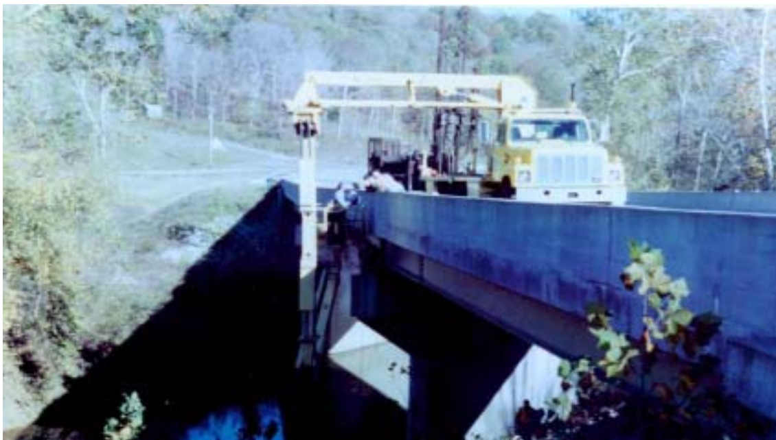
Figure 2-5: Installation of the junction box on pier No.2 of the S.R.62 bridge over the Little Blue River, Crawford County, IN.
