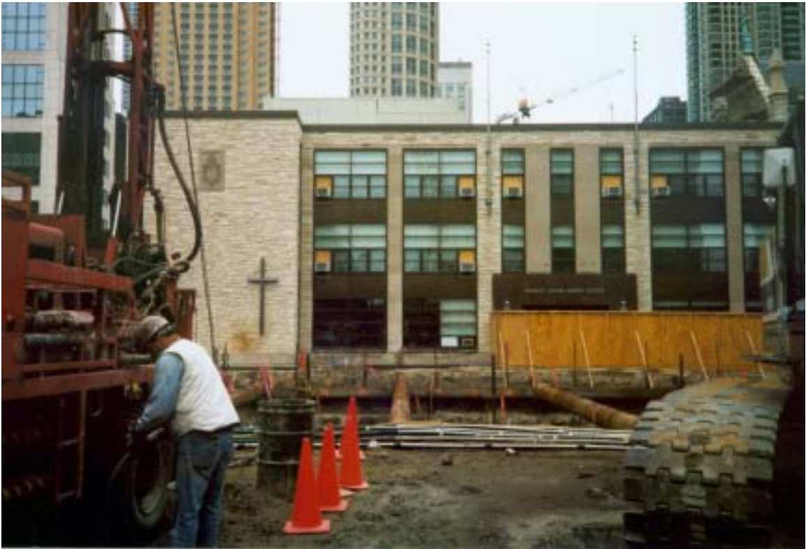
Figure 5-4: View of the drilling of TDR-1, Chicago & State subway excavation, Chicago, Illinois (the Frances Xavier Warde school is seen in the background).
