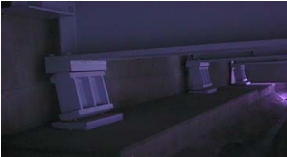
Figure 3-9: Rotated rockers bearings of the bridges on I-64 over the Little Blue river, Crawford County, Indiana.
