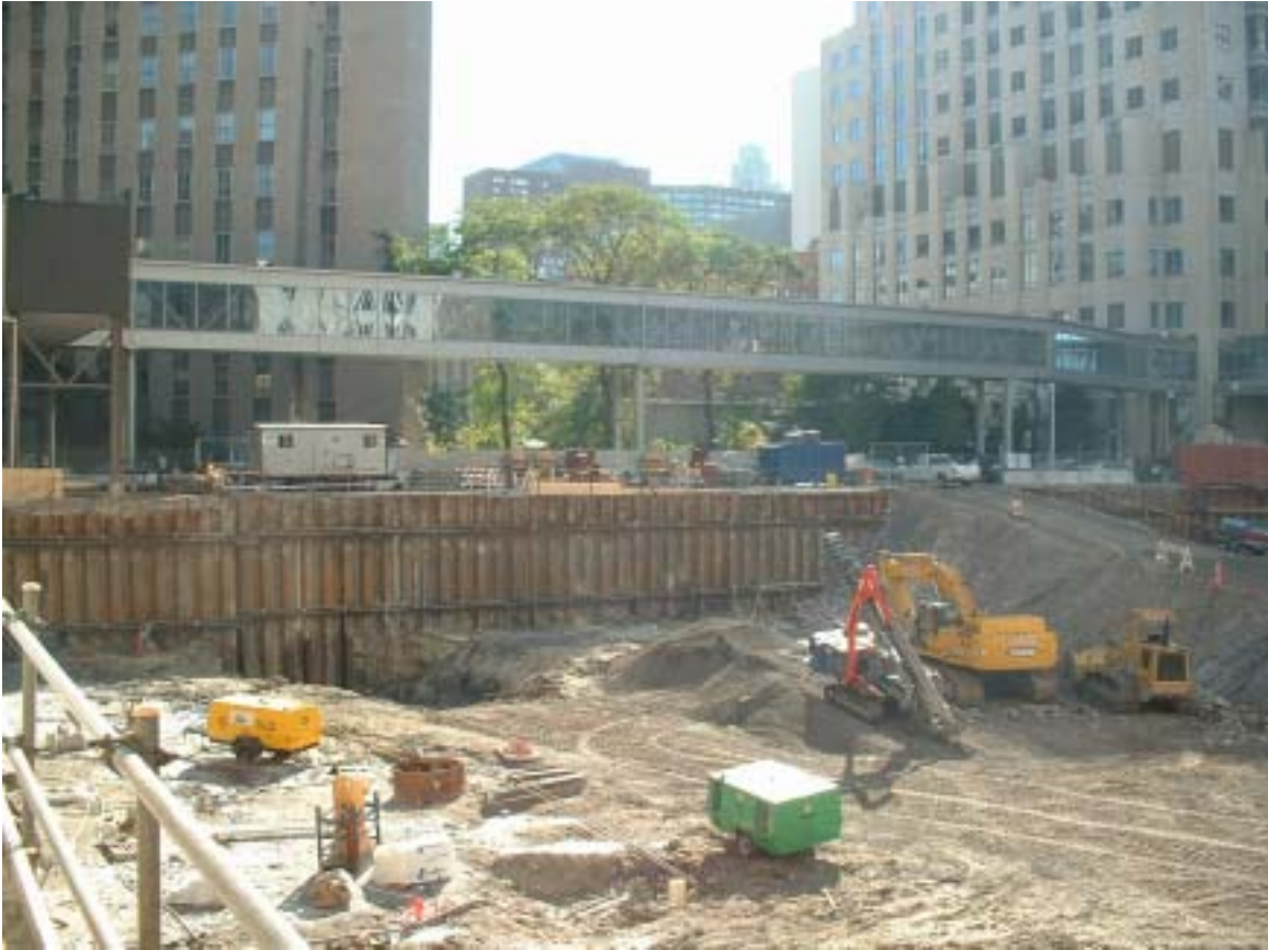
Figure 5-9: View of the south wall (Huron St.) of the Lurie Research Center excavation showing the first and second level of tiebacks, Chicago, Illinois.
