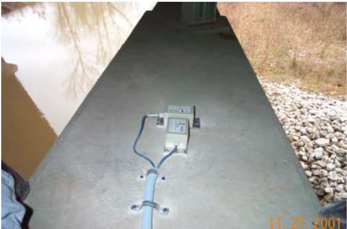
Figure 2-6: Installation of tiltmeters TL-1 and TL-2 over the centerline of pier No.2 of the S.R.62 bridge over the Little Blue River, Crawford County, IN.
