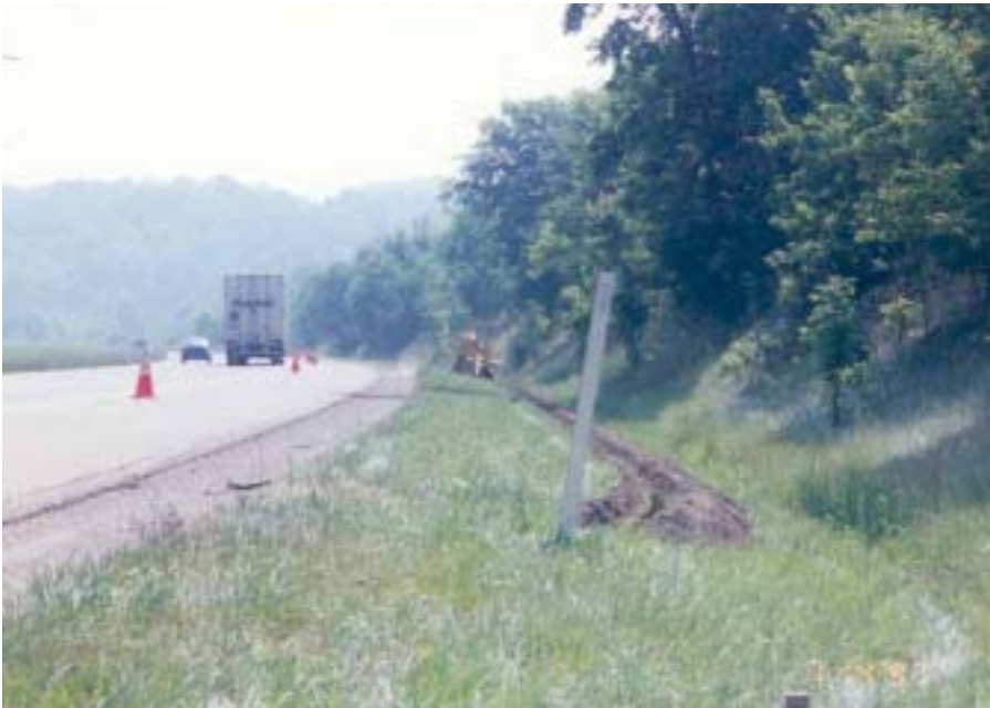
Figure 4-13: View of the Eastbound side of I-70, at point Mile 183.11 showing the trench for installation of transmission cable, Cambridge, Ohio
