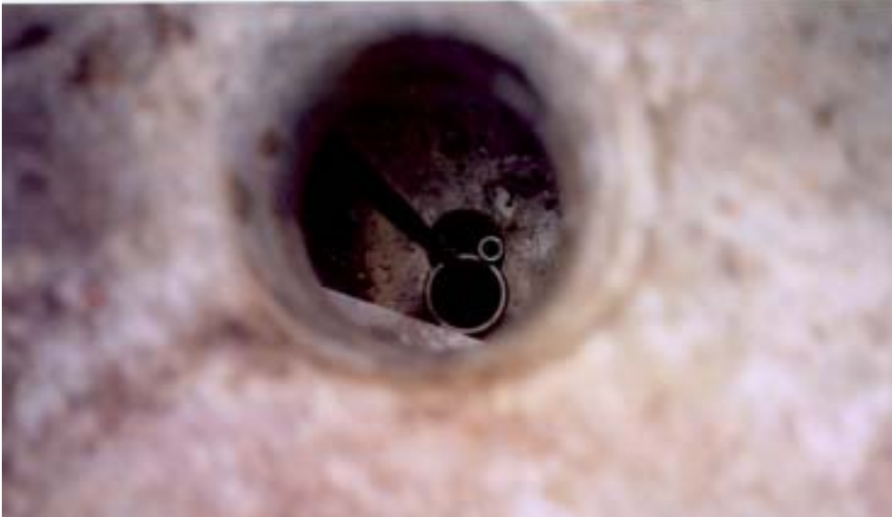
Figure 2-16: View of the 4 in. and 1 in. casings housing the TDR cables through the deck of bridge 02-117 over the Klamath River, Horse Creek, CA
