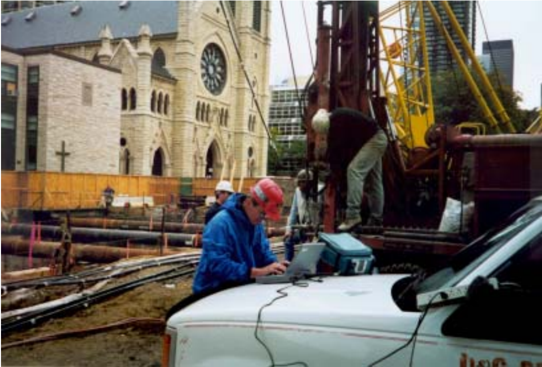
Figure 5-5: Kevin O'Connor (GeoTDR Inc.) is taking a manual reading on TDR-1 with a Tektronix 1502 pulser and a laptop computer, Chicago & State subway excavation, Chicago, Illinois.
