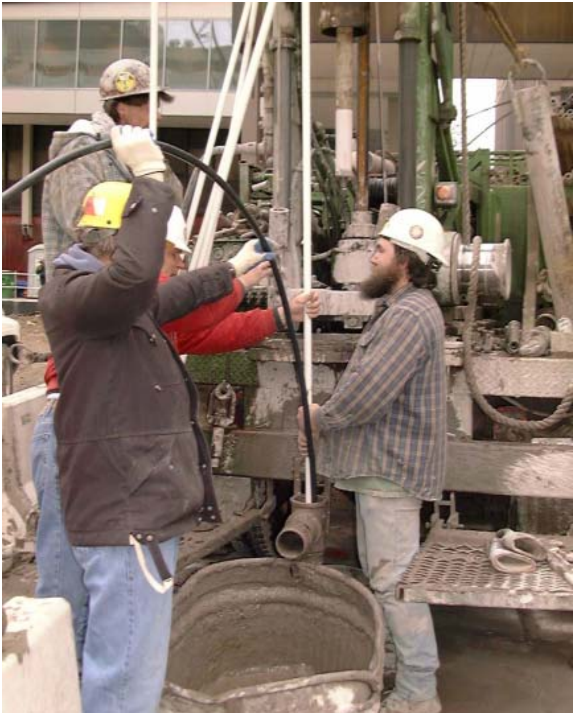
Flexible cable insertion with a cone attached to it and pushed down with a PVC pipe
