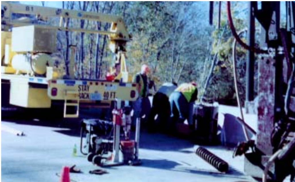
Figure 2-4: Drilling of hole TDR-2 from the deck of the S.R.62 bridge over the Little Blue River, Crawford County, IN.
