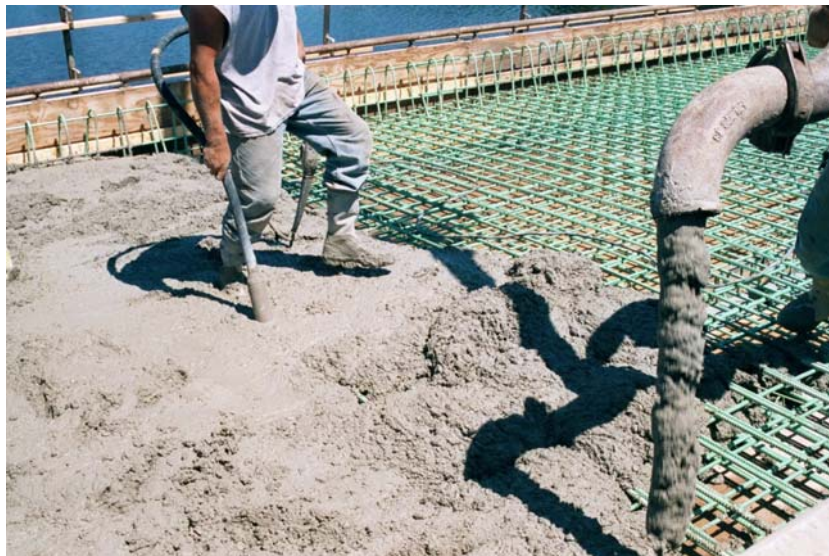
Figure 3-2: Fresh concrete being poured into a framework containing steel rebar. (Image courtesy of the Portland Cement Association).
