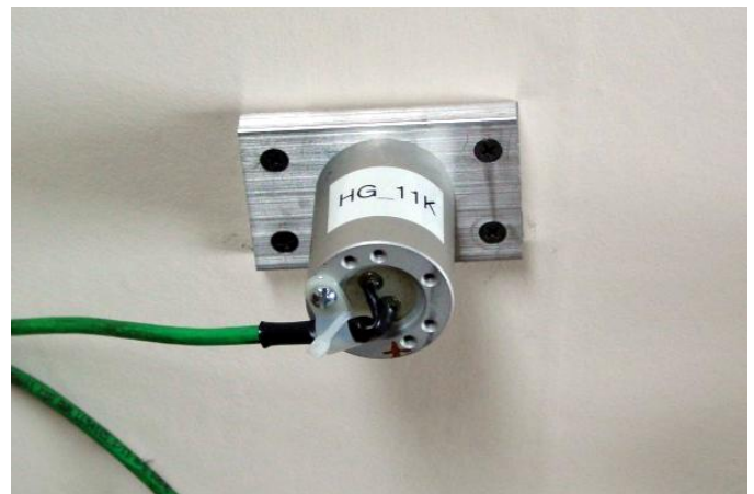
Figure 15: Vertical Geophone: Ceiling
