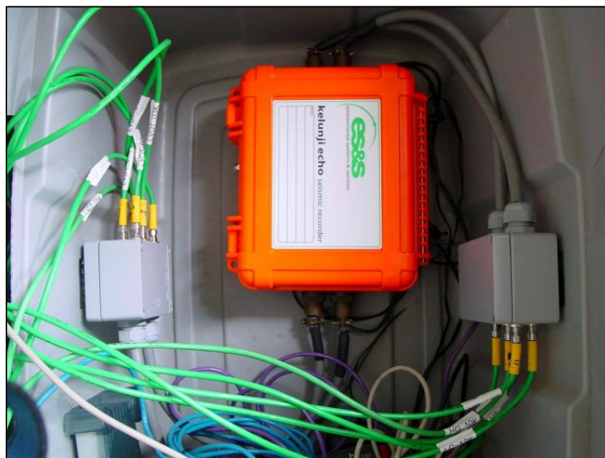
Figure 2: KEP and connector boxes in field container
