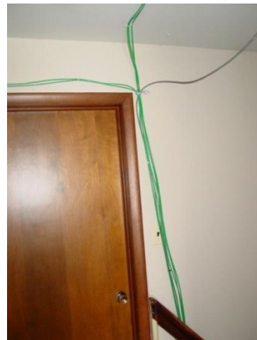
Figure 27: Example Wall Wiring
