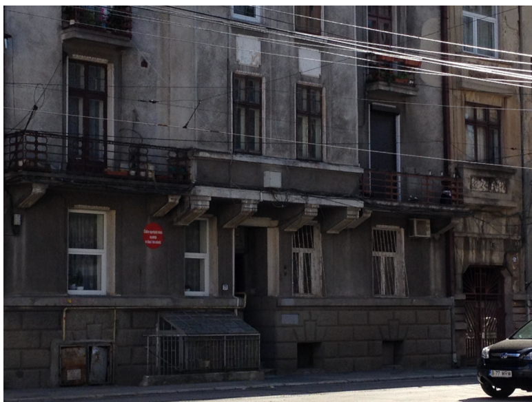
Figure 13. Apartment building in Bucharest with a prominent “red dot” indicating its assessment in Class I for seismic risk. 65
