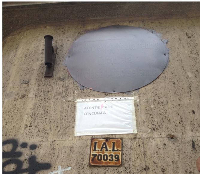
Figure 14. Painted over “red dot” Class I seismic risk sign above the handmade, home-printed sign in a plastic sleeve that states, “Attention, falling plaster.” 84
