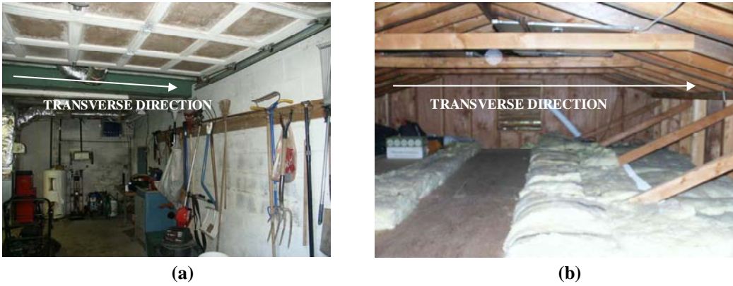
Figure 2.5 Photos of ceiling joist systems (a) garage ceiling/apartment floor system, (b) apartment addition ceiling truss system
