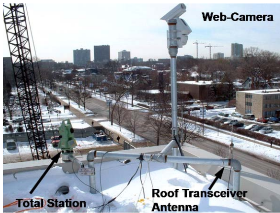
Figure 6: Total Station and webcam on rooftop of adjacent building.
